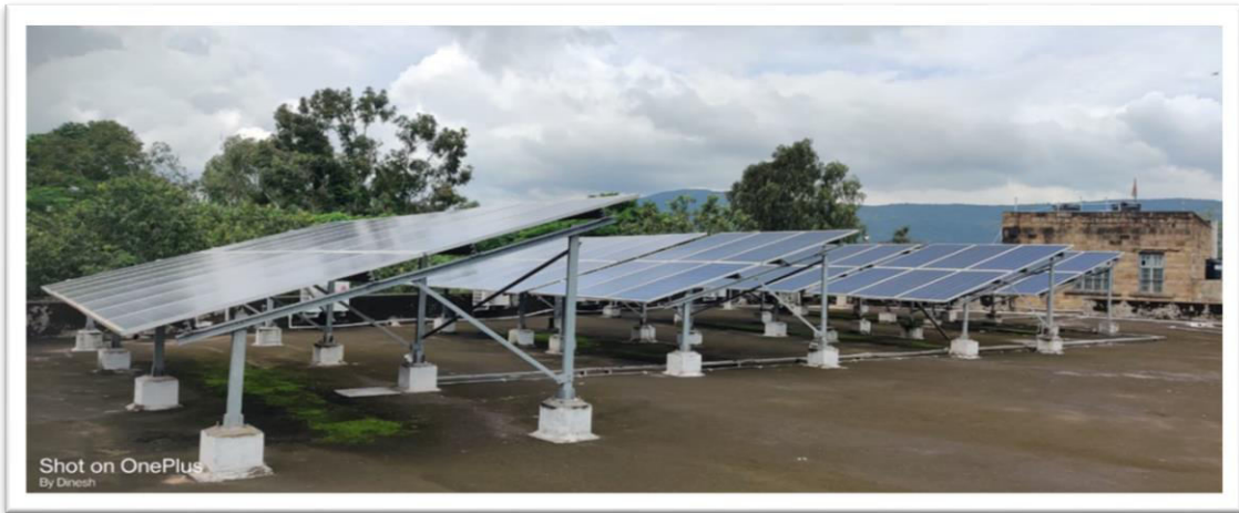
Renewable Energy on the roof top of Chemical Engineering Department
